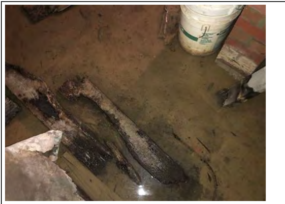
WATER IN BASEMENT OF SUBJECT PROPERTY
